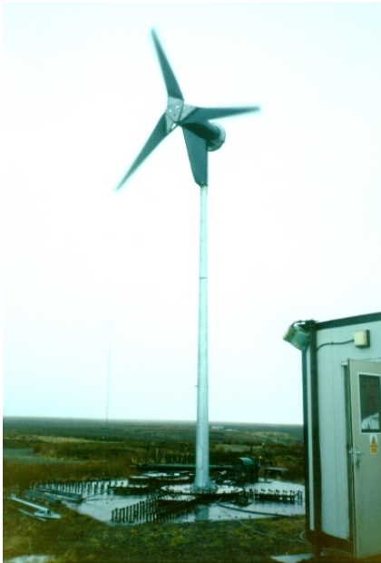
Figure 4: Proven turbine installed at NEL test site
