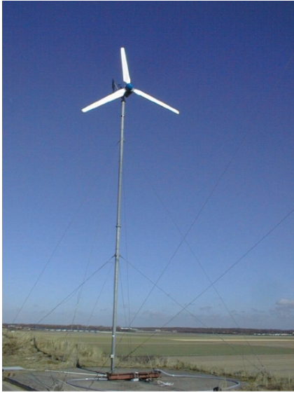
Figure 7: Fortis Montana Turbine at ECN test site
