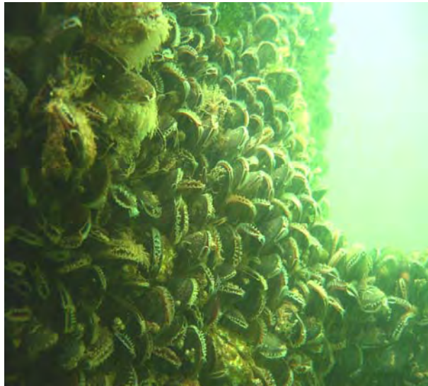
Figure 10: Mussel growth at foundation. Photo: EMU Ltd
