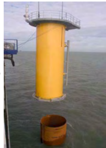
Figure 3: Installation of the transition piece onto the monopole foundation. Photo: Chris Laurens
